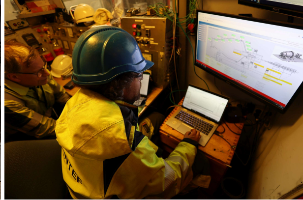
Figure 2. Control room of the rotary furnace
