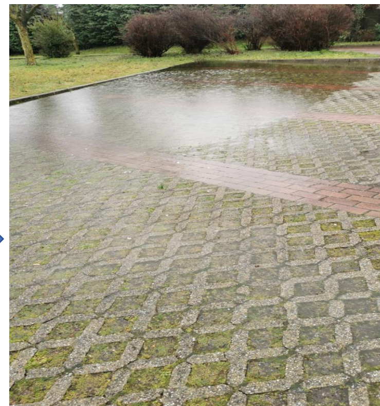
Even attempt to mitigate soil sealing not working
