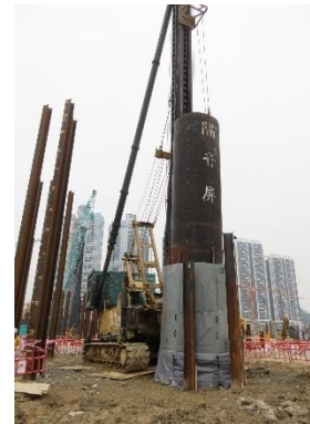
Figure 13: 5m (H) x 7m(L) SilentUP ® at Liantang / Heung Yuen Wai
