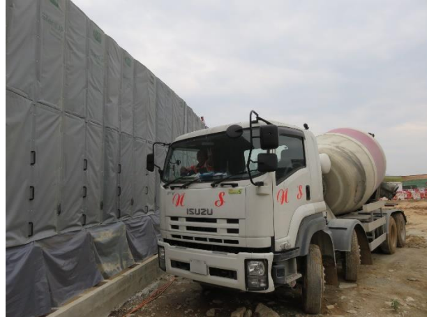
Figure 7: 5m (H) x 16m(L) SilentUP® at Liantang / Heung Yuen Wai
