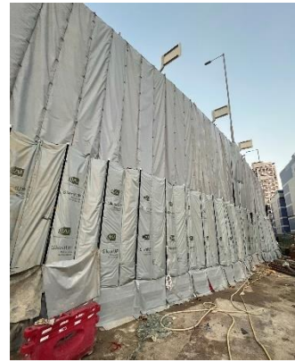
Figure 17: 7m (H) x 38m(L) x 33m(W) SilentUP ® at Central Kowloon Route
