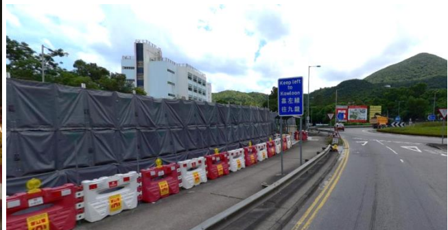
Figure 9: 3m (H) x 55m(L) SilentUP® at Hiram's Highway
