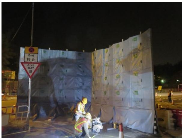
Figure 8: 5m (H) x 11m(L) SilentUP® at Castle Peak Road
