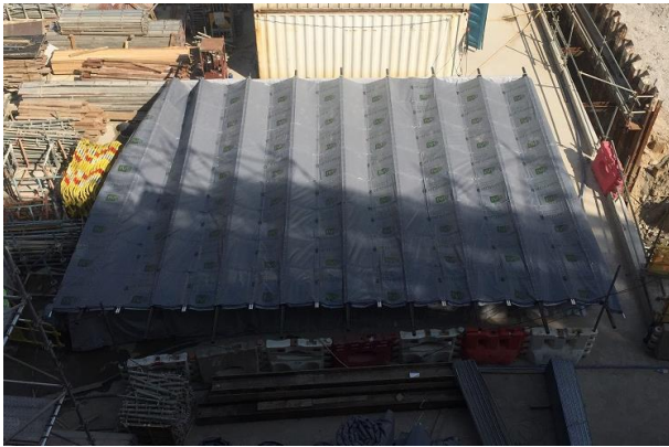
Figure 16: 8m (W) x 11m(L) SilentUP ® at Hong Kong West Kowloon Station
