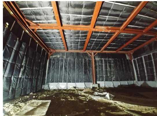
Figure 19: 7m (H) x 18m(L) x 15m(W) SilentUP ® at Central Kowloon Route
