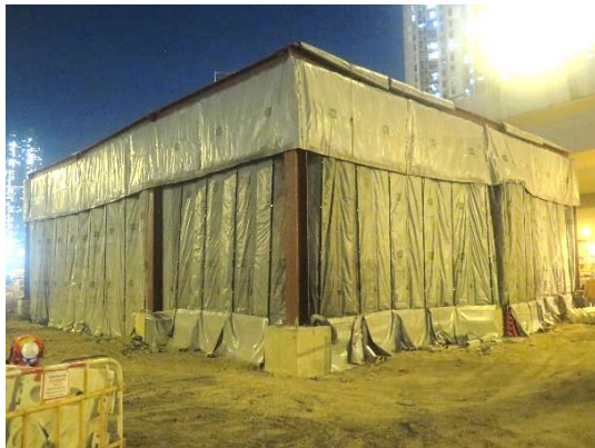
Figure 18: 7m (H) x 18m(L) x 15m(W) SilentUP ® at Central Kowloon Route
