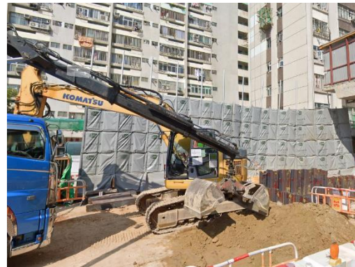
Figure 11: 5m (H) x 16m(L) SilentUP ® at Castle Peak Road
