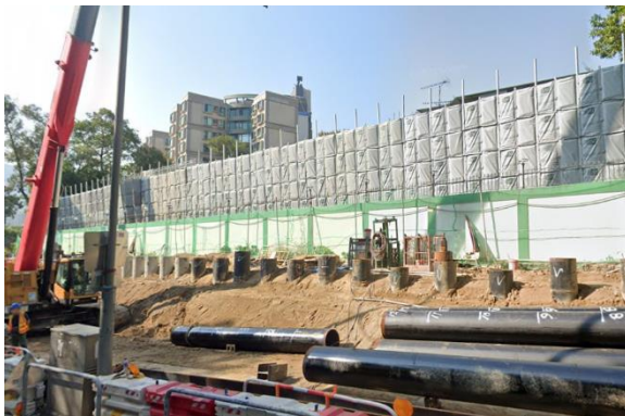
Figure 12: 5m (H) x 50m(L) SilentUP ® at Castle Peak Road
