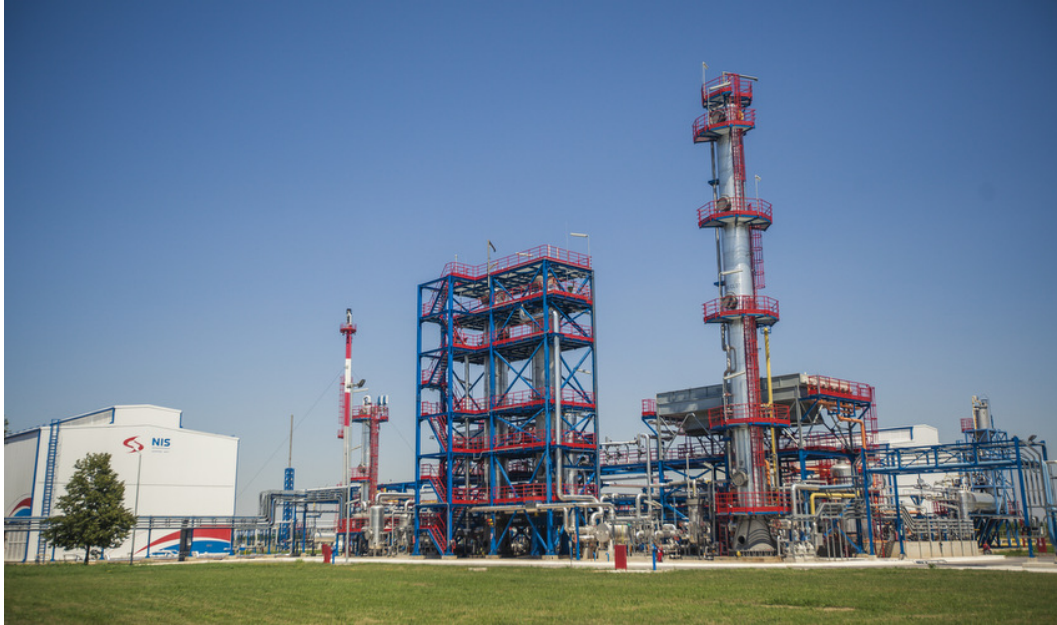
Figure 1 The HiPACT™ plant in Elemir, part of the gas processing plant
