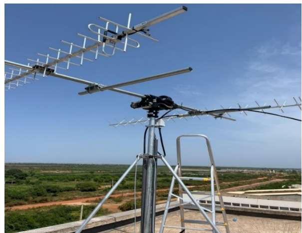
Figure 11: Antenna of the ground segment
