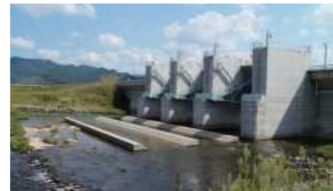
Hwasoon Flood Control Center
