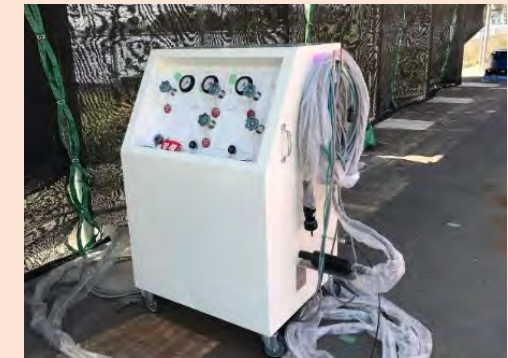
Class 2 high pressure gas Manufacturing facility
