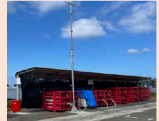
Class 2 high pressure gas storage facility (cardle storage)
