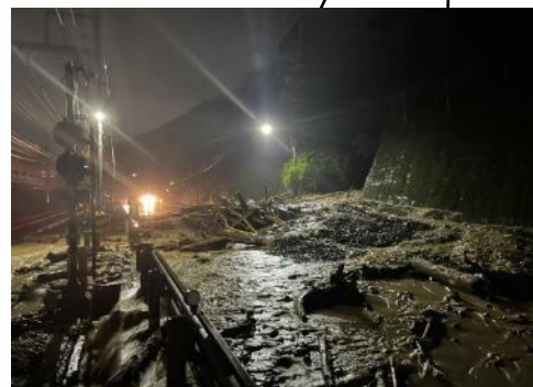
Damaged National Highway Route 1 (Closed for 4days & 7hours due to landslide)
