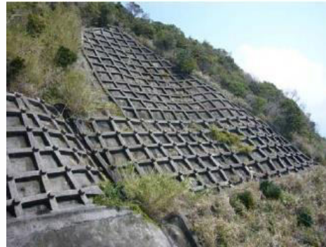
Slope protection with concrete frame and stabilization anchor
