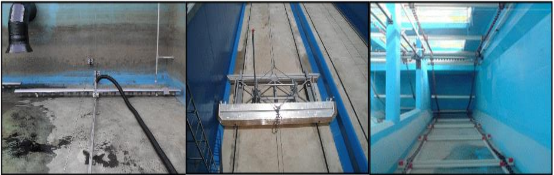
● Existing sludge collector
