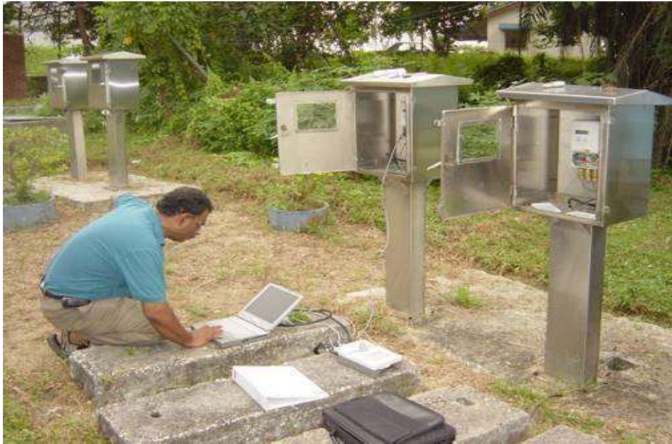
Yearly electronic verification of Bulk Meters
