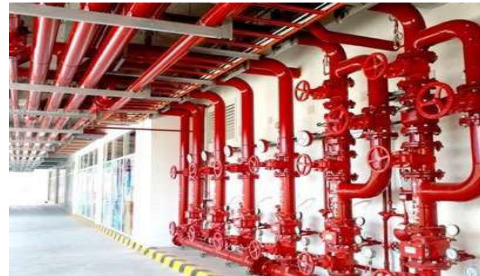
Fire fighting requirements critical to pressure management
