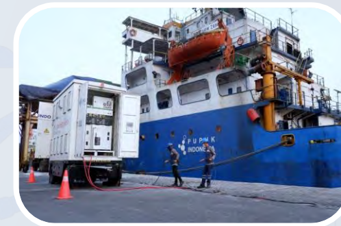
On Shore Power Supply
