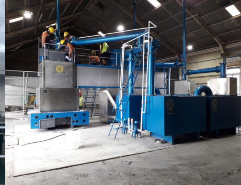
ELECTRIC INCINERATOR AT SUVA PORT
