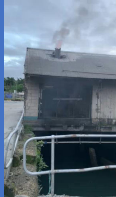
OLD DIESEL INCINERATOR
