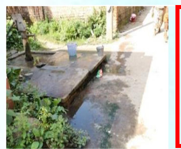
Lack of LWM
