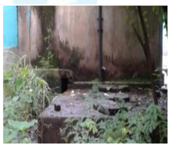
Poor Sanitary Condition
