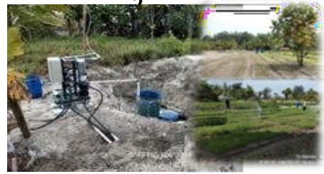
Type-1 (AC Pump, Bulk Irrigation)
