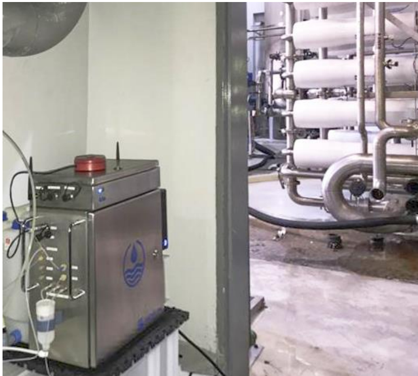
THE COLIMINDER INSTALLED FOR MONITORING DRINKING WATER BOTTLING IN SOUTH AFRICA
