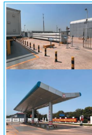
Hydrogen fuel at Qingdao Port. Pictured above are pipes for pumping the hydrogen fuel into trucks, a refueling station (photo by Nestra).
