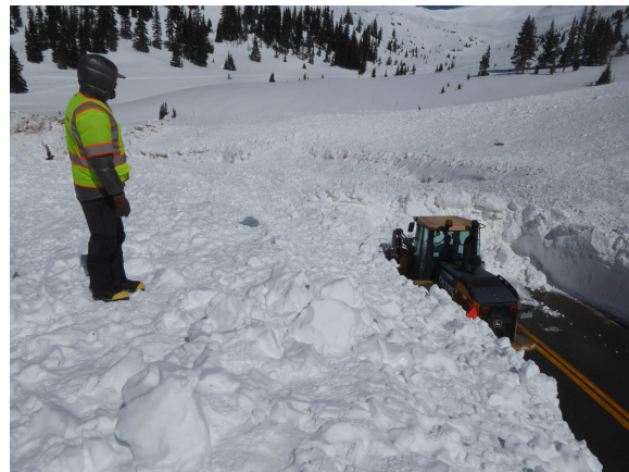
Figure 2. An example of an intolerable event. Large avalanches can require heavy equipment to clear the debris from the roadway, resulting in unusually long closure times that can quickly cause traffic delays and loss of revenue.
