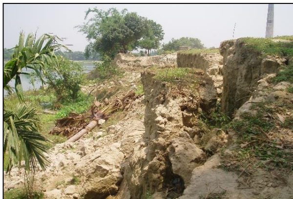
Figure 2. Subsidence occurred in Kapasia-Sripur road
