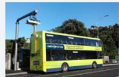
Battery electric bus charging infrastructure
