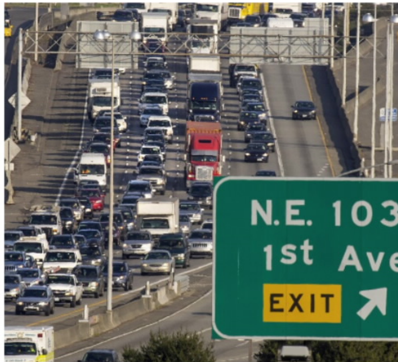
1 of 2 A 2015 emergency-repair job on an Interstate 5 South expansion joint near the West Seattle exit clogged traffic through Seattle with backups reaching 13 miles north of the repair site. This view looks north from... (Mike Siegel/The Seattle Times) More ▾
