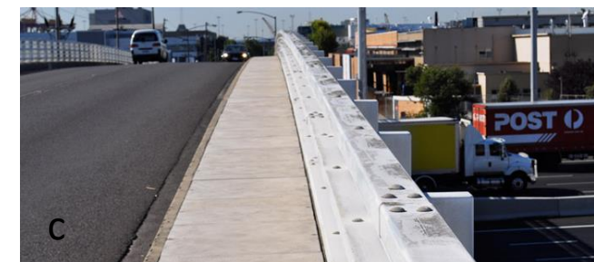
Figure 4. Examples of E-Crete in Australia: (a) in-situ retaining wall, (b) freeway, (c) precast bridge panels, Zeobond Pty. Ltd., ( http://www.zeobond.com/ ).
