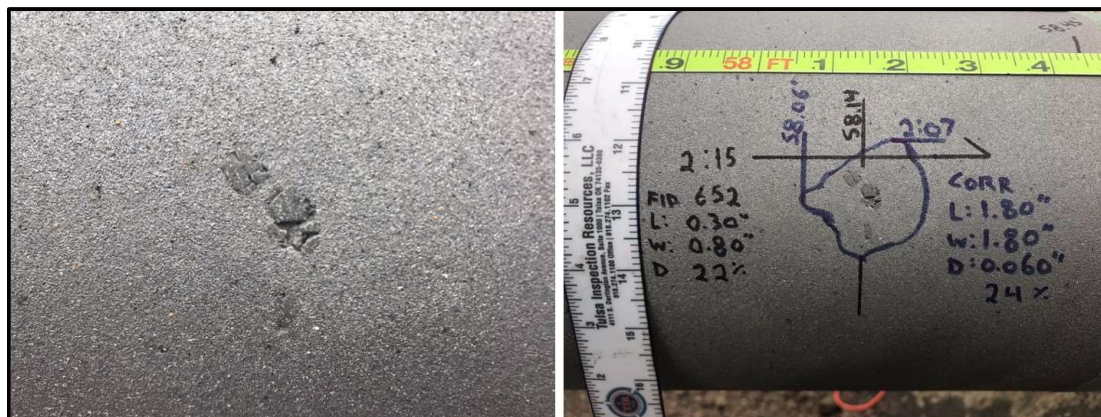
Figure 2 - Pipe mark-ups can make a difference
